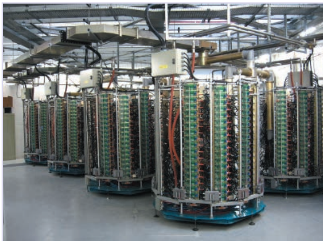
Figure 3.1.10: 8 x 50 kW solid-state power amplifier towers operated at SOLEIL, combining the power from 300 W modules with LDMOS-FET transistors in push-pull configuration. Such solid-state high power technology has been shown to provide a more stable system and is expected to have a longer lifetime than klystrons. It is planned to develop it for the ESRF in order to replace the klystron transmitters.
