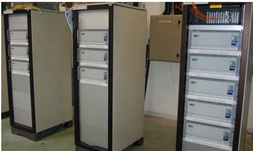
Figure 4.9: One quarter of the Bilt power supplies for AC steerers driven by the Fast Orbit Feed Back.
