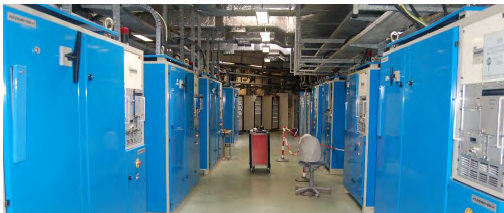
Figure 4.6: SRDC room with future refurbished AC/DC rectifiers.
