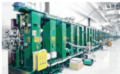
"SAES GP500 MK5 NEG pumps installed on the in-vacuum undulator (NEOMAX)"
